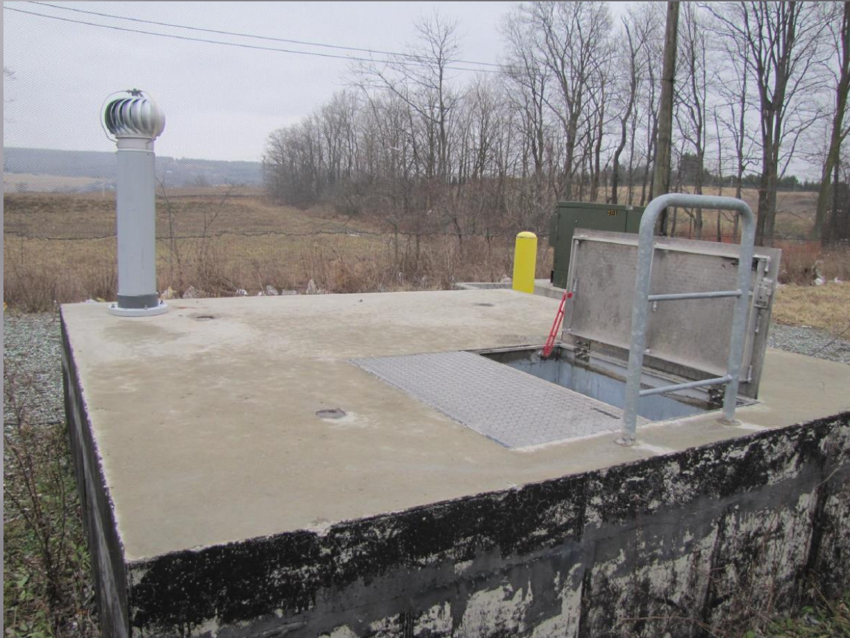
Vault for cleanout or wet well
