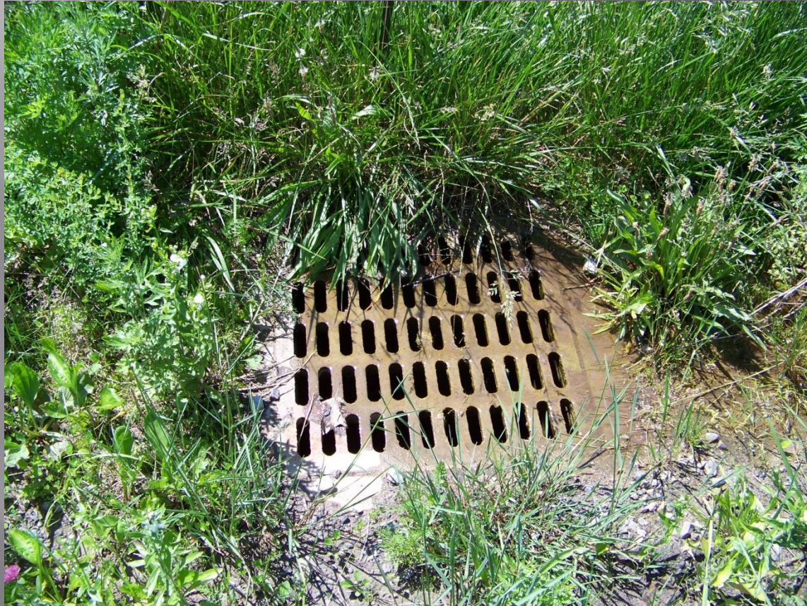
Storm Water Catch Basin
