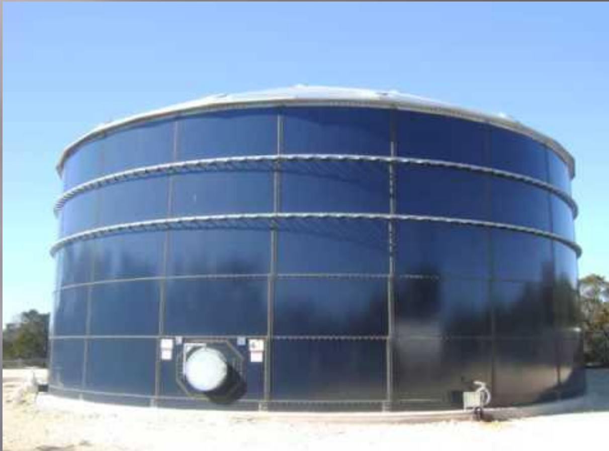
Leachate Storage Tank
