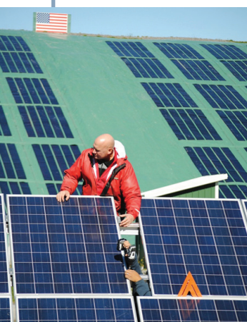
New solar panels were installed at the Madison County Landfill in front of the 40 kW photovoltaic membrane; both arrays provide significant cost savings for the Department of Solid Waste.
